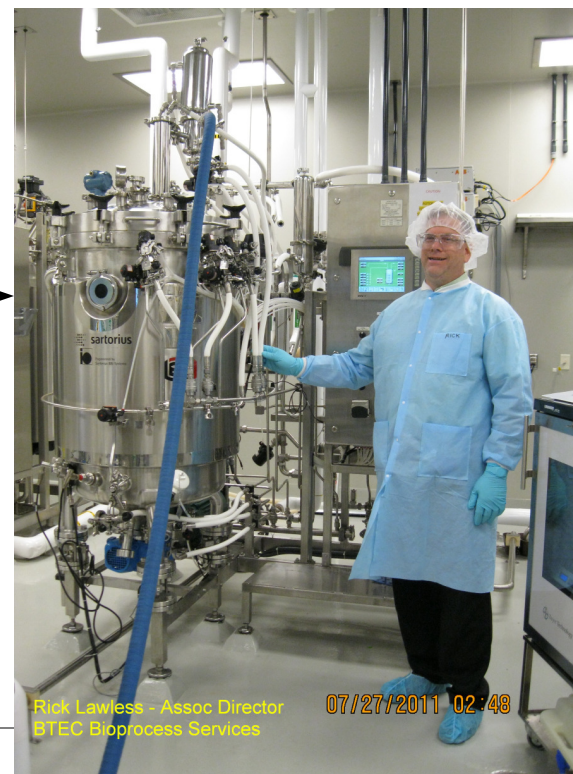
BTEC 300 liter reactor
